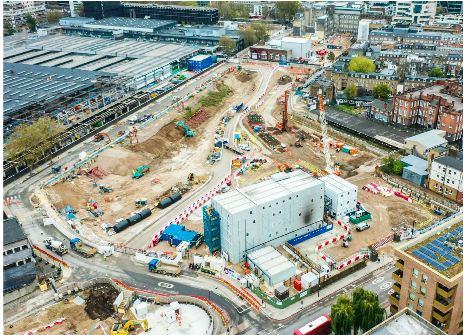
Aerial photograph of the HS2 Euston construction site and former Maria Fidelis school site
