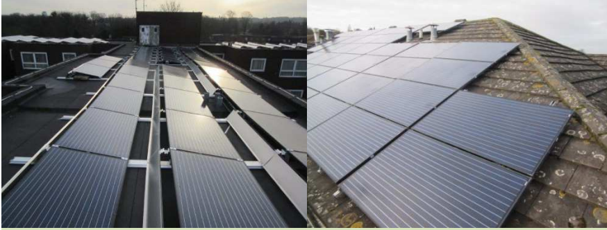
(Image: Solar PV panels on the roofs of Little Heath and Mandela House, installed in February 2016)
